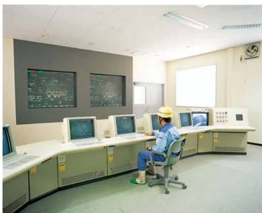
Utility Monitoring Center
