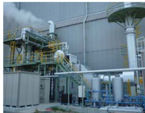
Exhaust heat recovering boiler
