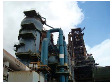
No.12 hot-blast stove
